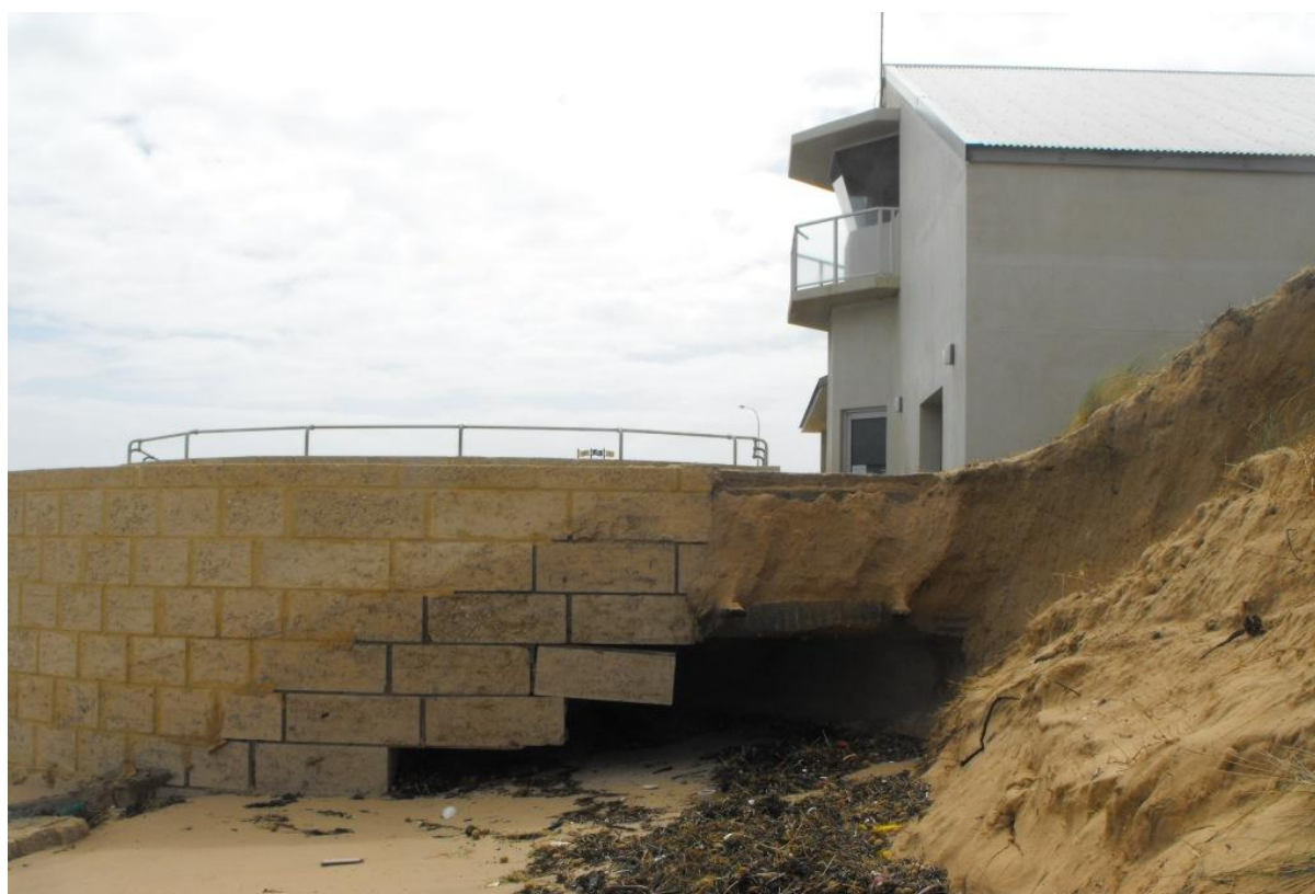
Figure 6-16: Exposure of Seawall Southern End Following September 2013 Storm
