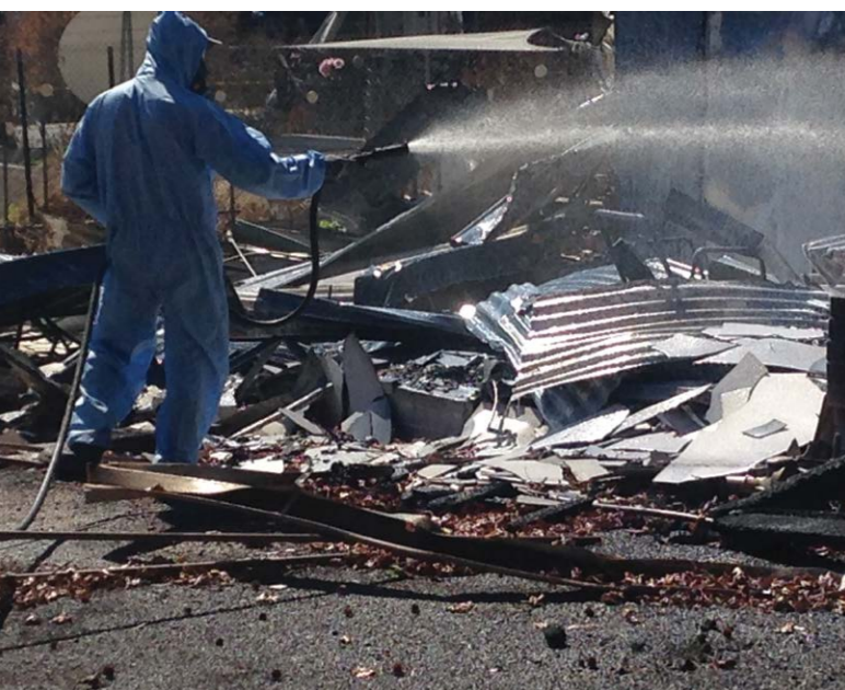
Clean up crews clearing Yarloop of asbestos and PCB contamination. Photo courtesy of Haydn Jones
