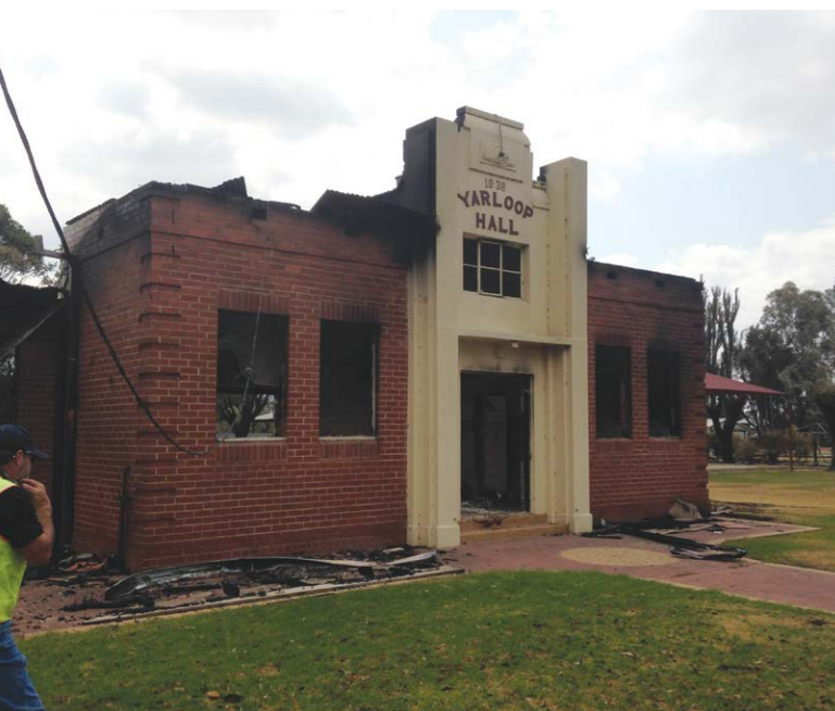
The fire-scarred shell of the Yarloop Hall. Photo courtesy of Haydn Jones
